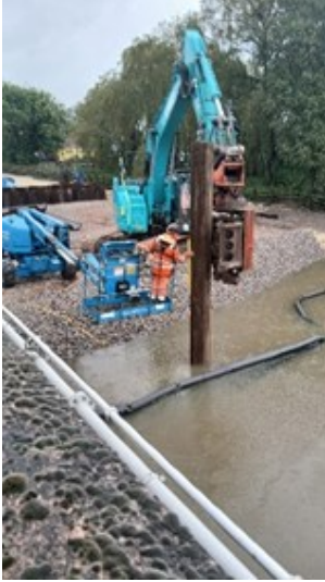
Sheet Piling on the east side of the river to create a cofferdam for the east pier base.
