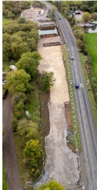
Zouch Bridge looking towards the A6 from Zouch village. Aerial view shows the route of the east approach road in the foreground
