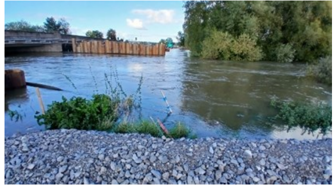
View of the east pier base, looking from the west side of the river across to the east side.
